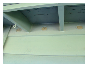
Plugged Attic Intake Vents
