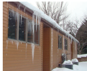
Ice Damming Problems
