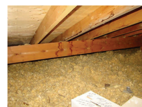
Evidence of Condensation
